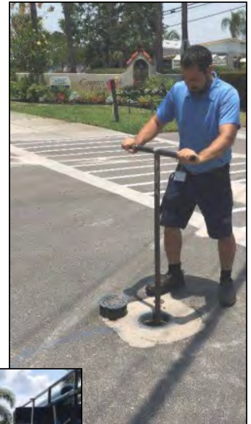
Above, Vadim Bugayev exercises valves on Golf Dr., part of the Water Main Replacement Project Phase 5. At left, Derek Selk and Hans Ferjuste inspect blowoffs and conduct chlorine tests in Venetian Golf & River Club.
